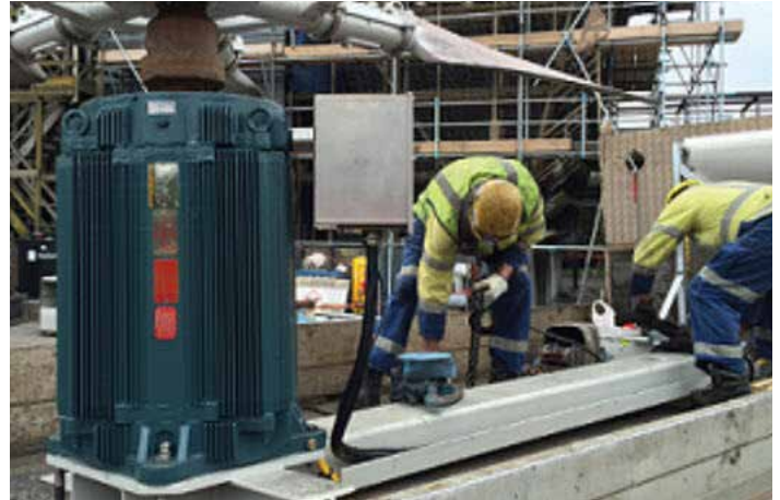
On-site commissioning, repair, and predictive and preventive maintenance for motors and generators
