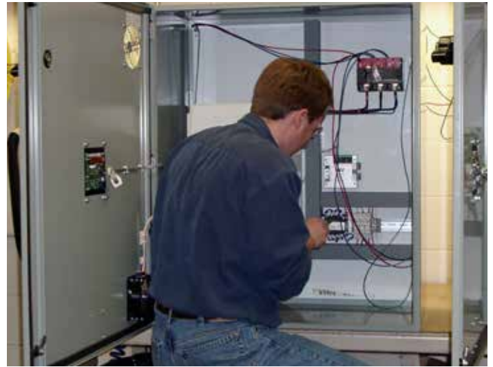
IPS engineering can help modify control panel operations for specific requirements.
