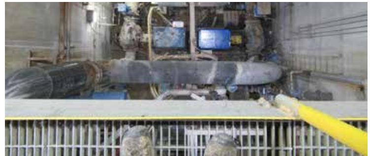
Limited space forced the customer to utilize WPI motors in a wet and harsh environment.
