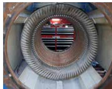
Motor with PowerSeal rewind after removal.
